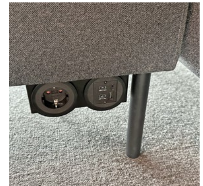
Power outlet under sofa
