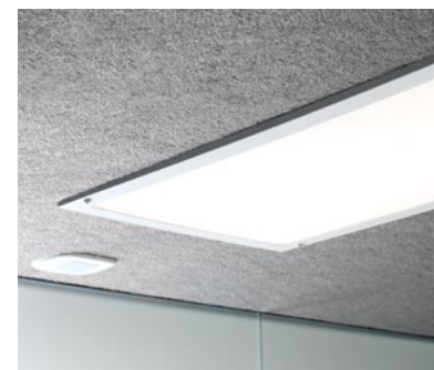
LED light with presence sensor
